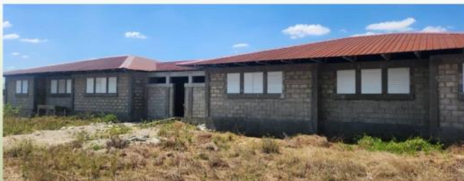
The initial structures on the Model Campus, including the residence buildings that will house missionary volunteers and LCS staff, are complete.
