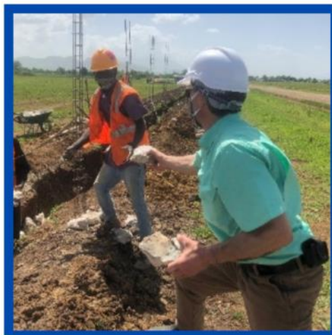
► June 2021: THP Director of New School Construction Jimi Grondin assists in placing the first stones in the foundation of the perimeter wall.
