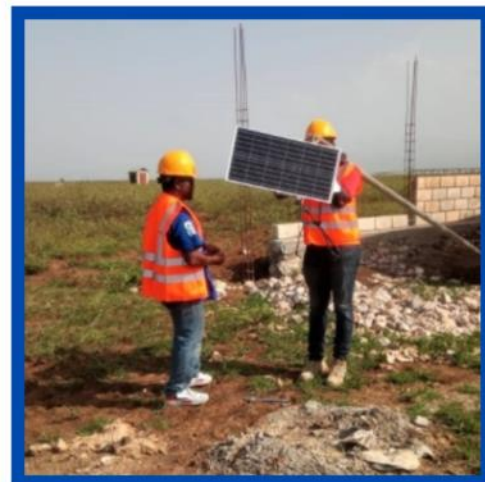
► September 2021: Workers install solar-powered lights to illuminate the grounds at the site.
