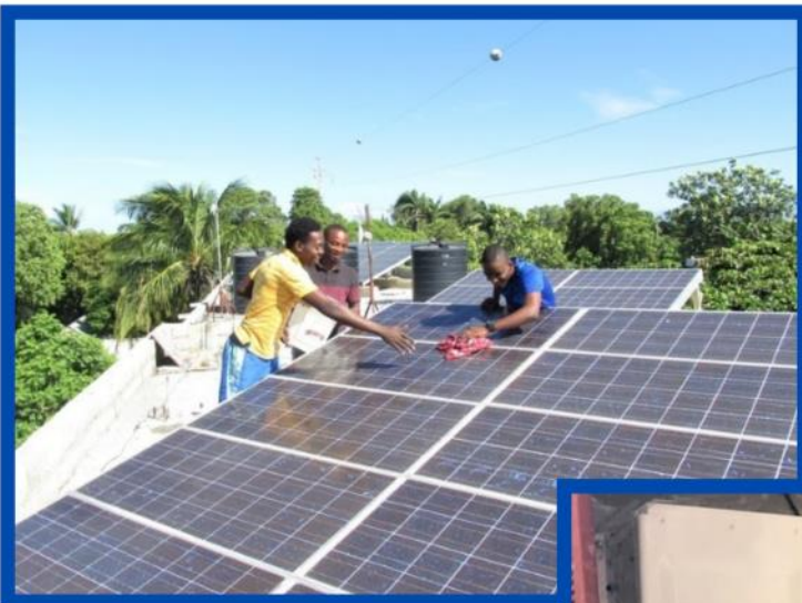
Louverture Cleary junior staff and students cleaning and maintaining solar panels on the LCS campus
